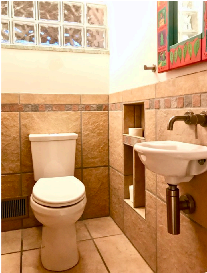
4395 Toilet Leak © 2019 Jesse Kumin
